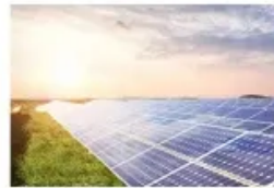
Energy Storage System
